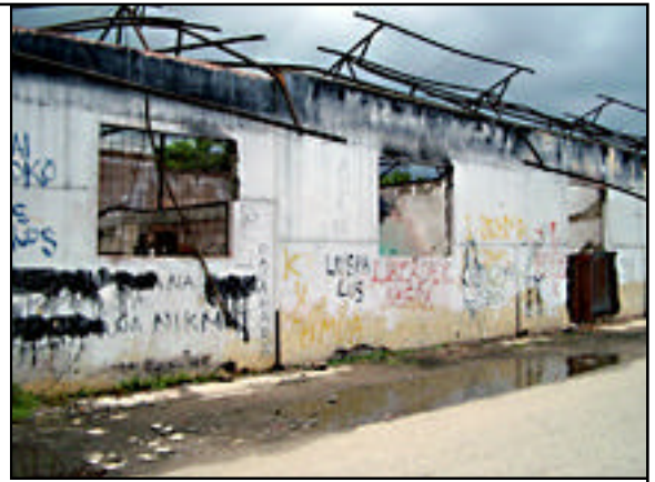
Buildings destroyed during clashes between Timorese nationals and anti-independence militias still stand in Dili.
